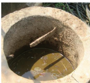
Rain (roof) water harvesting
