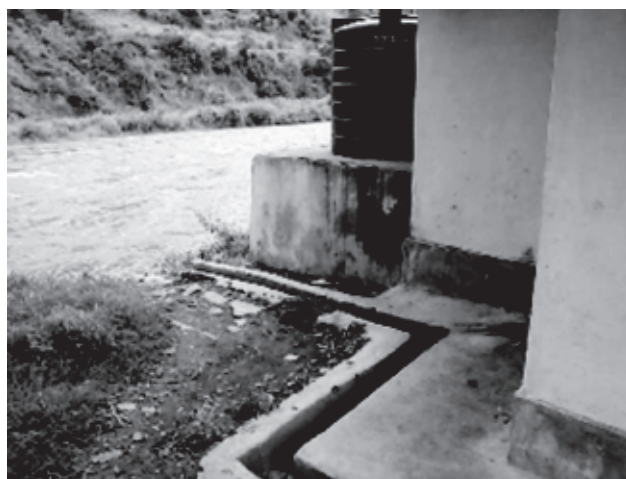
Photo 11.2 Drainage from public toilet
